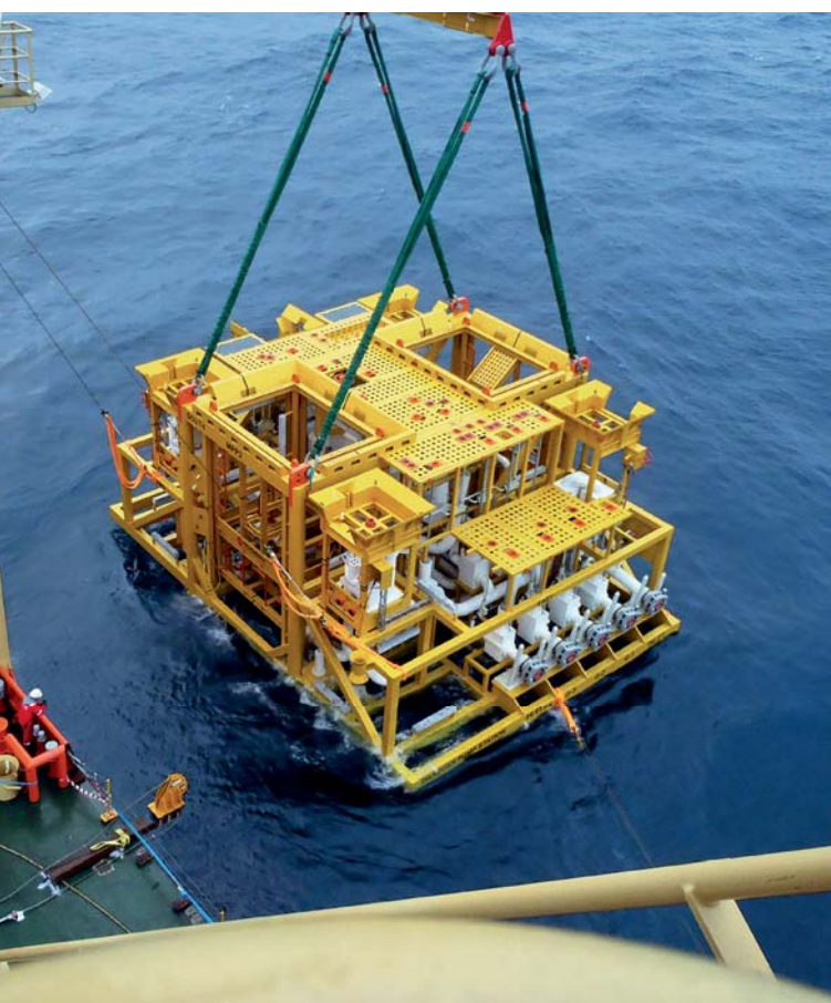
View of a multiphase subsea pump installation in the Shell Draugen field in the North Sea. The system integration of Framo pumps represented the world's first commercial subsea multiphase pump installation.
