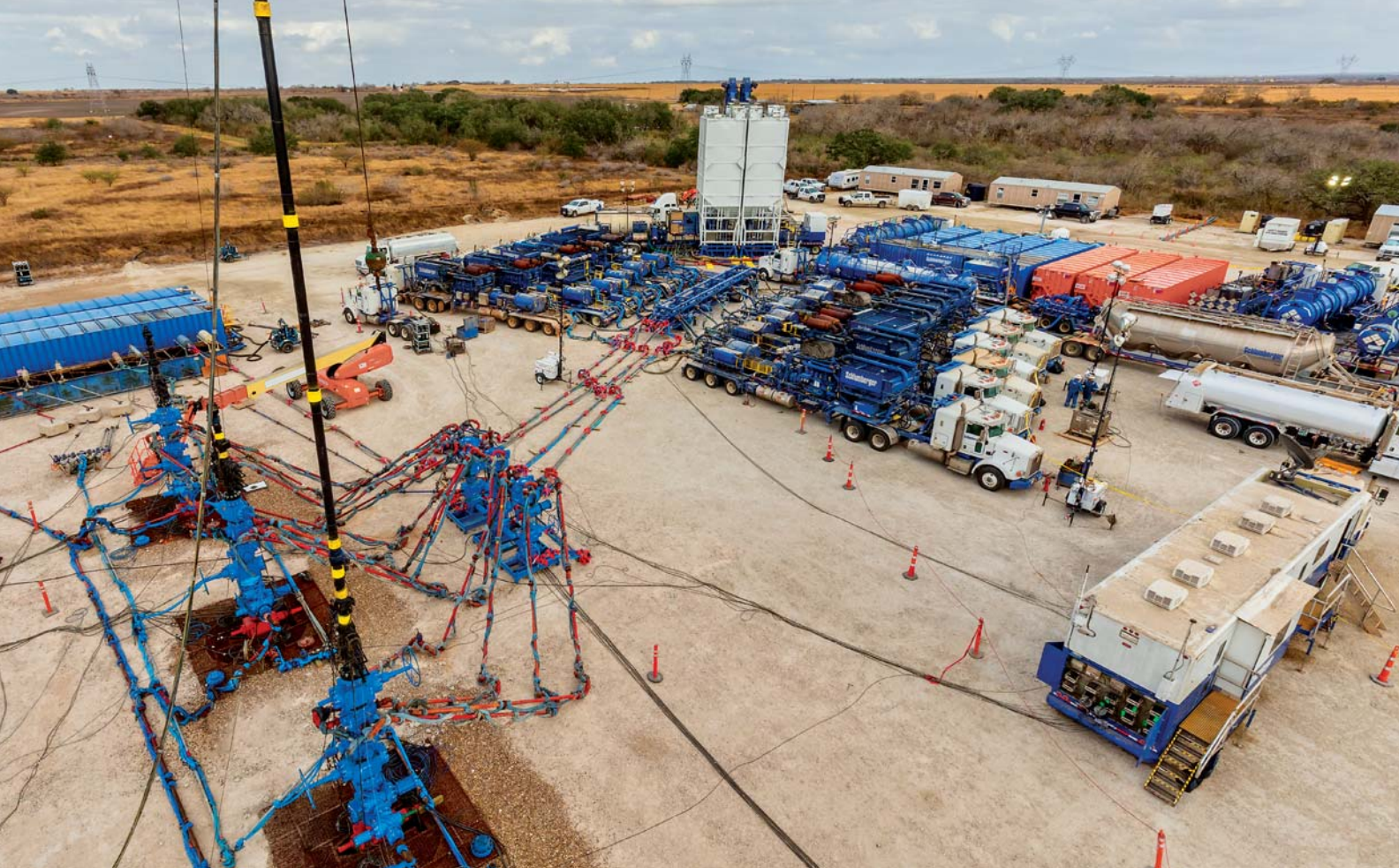
View of an integrated completions system operating in the Eagle Ford Shale basin. The combination of an automated stimulation delivery platform with fluid delivery and flowback services delivers hydraulic fracturing fluid to the wellbore, including fluid flowback and any subsequent well testing operations.
